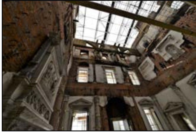
The Marble Hall after the 2015 fire.
